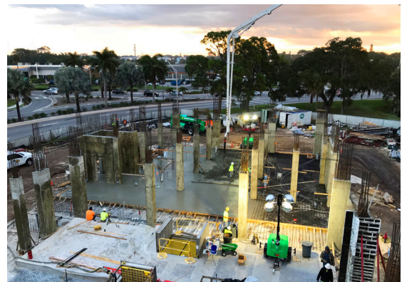
Crews worked 50 feet underground for more than a year to build the concrete wetwell for Lift Station 87. In August 2019, crews began work on the above-ground portion of the two-story brick lift station building.
